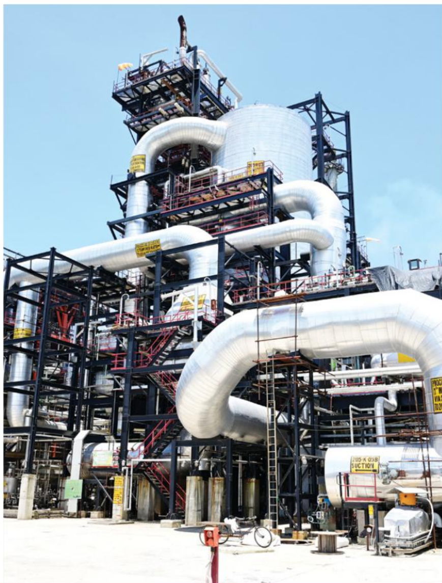
Wet Sulphuric Acid Plant at Haldia Refinery
