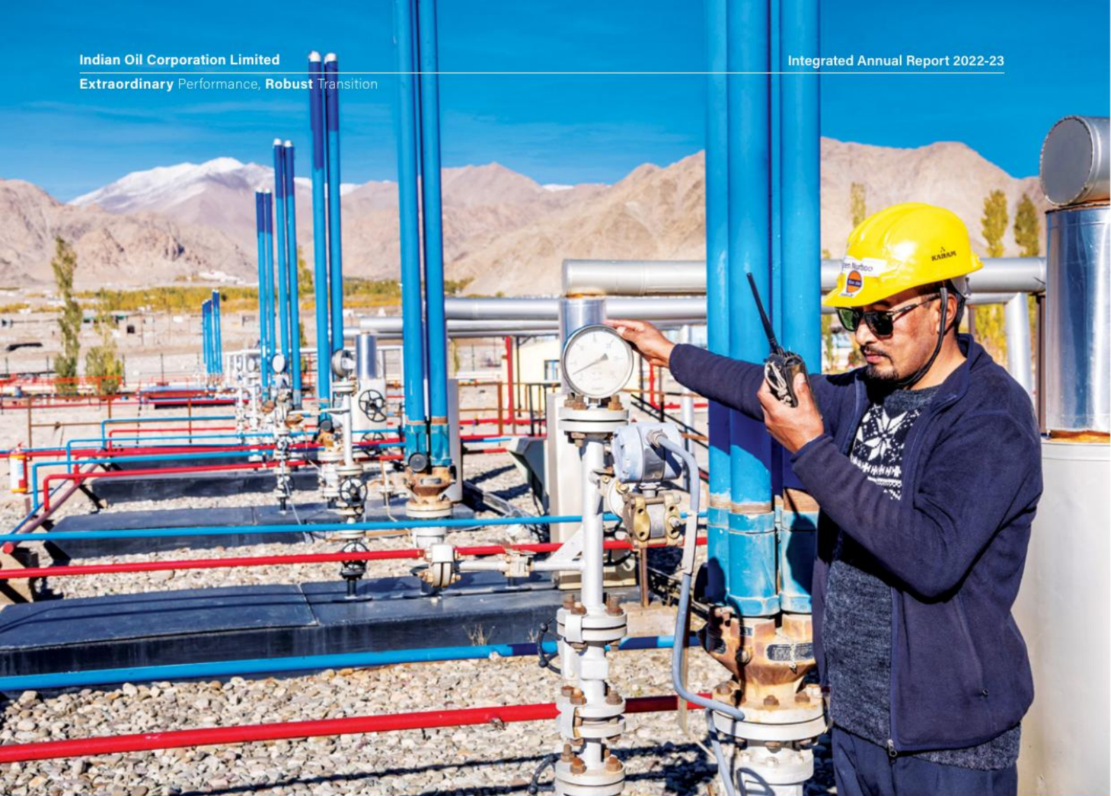
Product pipelines at Leh
